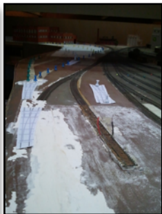
We had track in this portion of Bakersfield, but it was in such bad condition we couldn't run over it, so it has been torn out and is being replaced. The pins trace out the path the rails will follow
