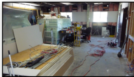
Meeting room last Fall with library books stacked, sheetrock and electrical supplies.— photos by Jeff Rowe, Dave Illich, Walt Freedman.
